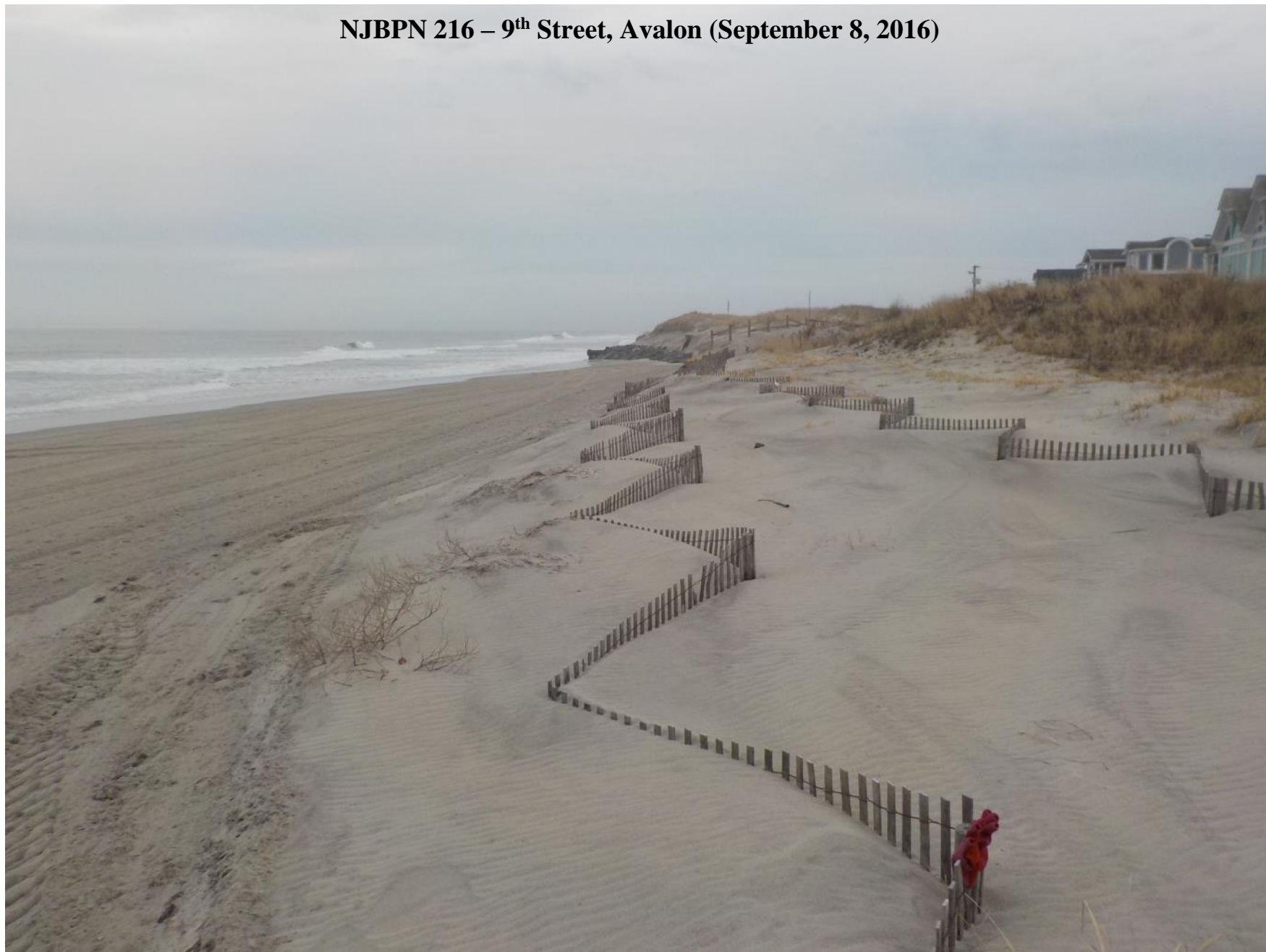
Figure 524. Two rows of sand fencing lie buried in sand placed by the Borough, yet beach erosion still reached the rock revetment at 12 th Street.
