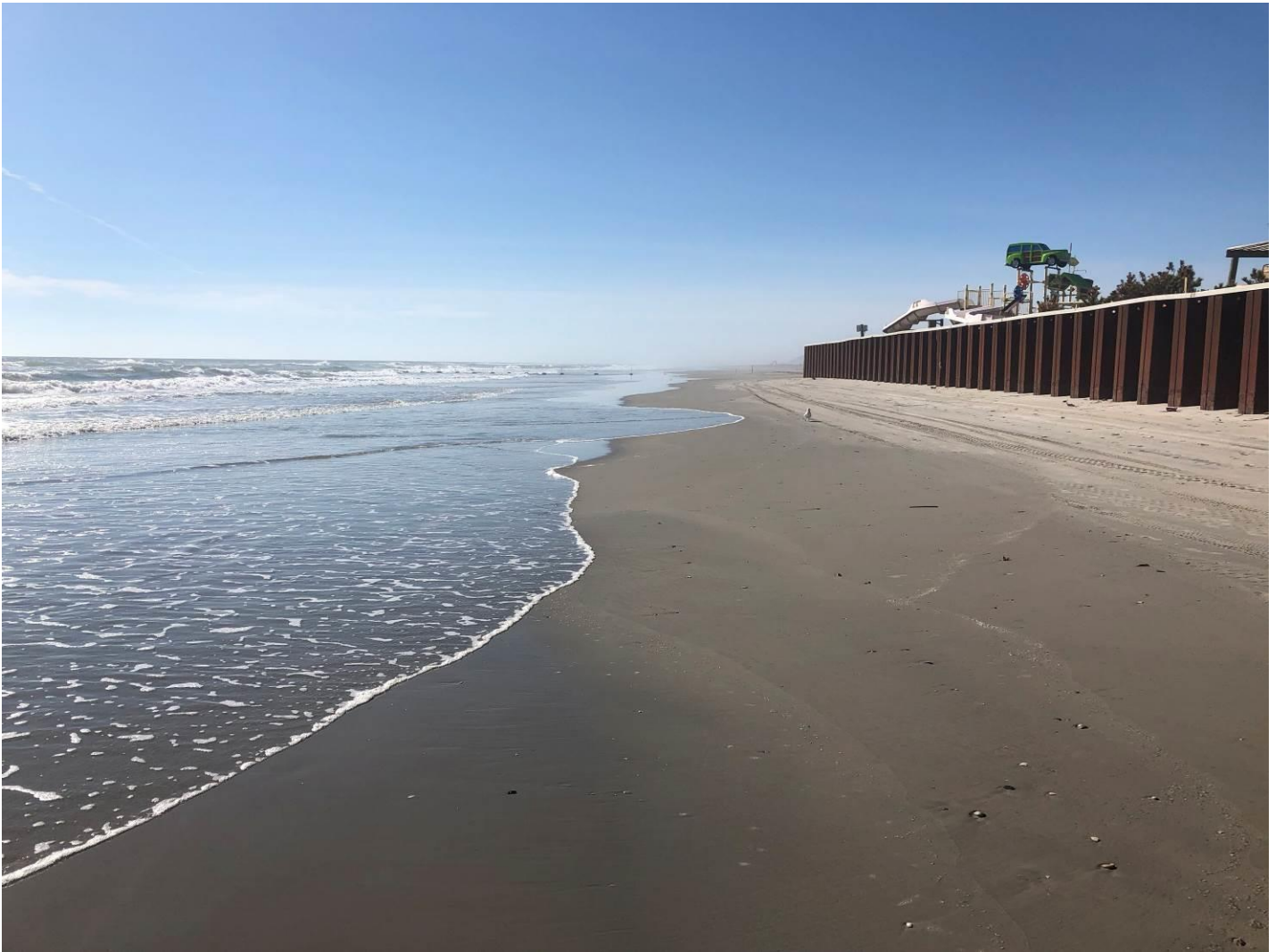
Figure 27. View to the south taken on November 11, 2018 near 26 th Avenue showing the beach at the Surfside Pier's seaward end steel bulkhead. Waves easily reach the bulkhead making a dry berm unlikely until the shoreline advances about 100 feet further seaward. Little change has occurred at the bulkhead in over a year with summer accumulations allowing minor beach use immediately seaward of the steel wall.
