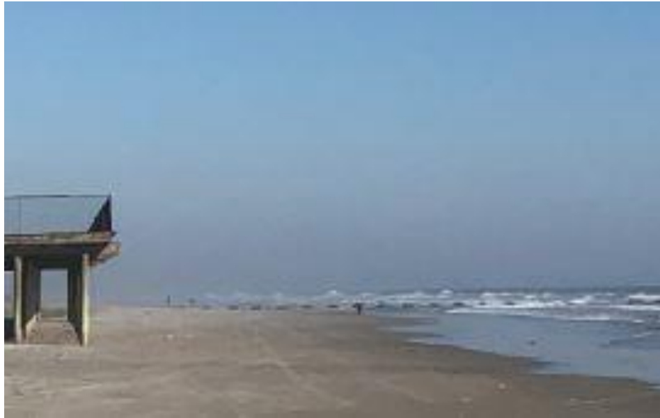
Figure 23. A close up view of the beach at the very seaward end of the timber pier indicating that no dry beach or dune feature remains at the pier's end (November 11, 2018). The dune extends to the pier and in between it and Morey's Surfside pier utilizing an older island dune existing on beach raking debris from years ago. This was essentially the same configuration the beach presented a year ago.
