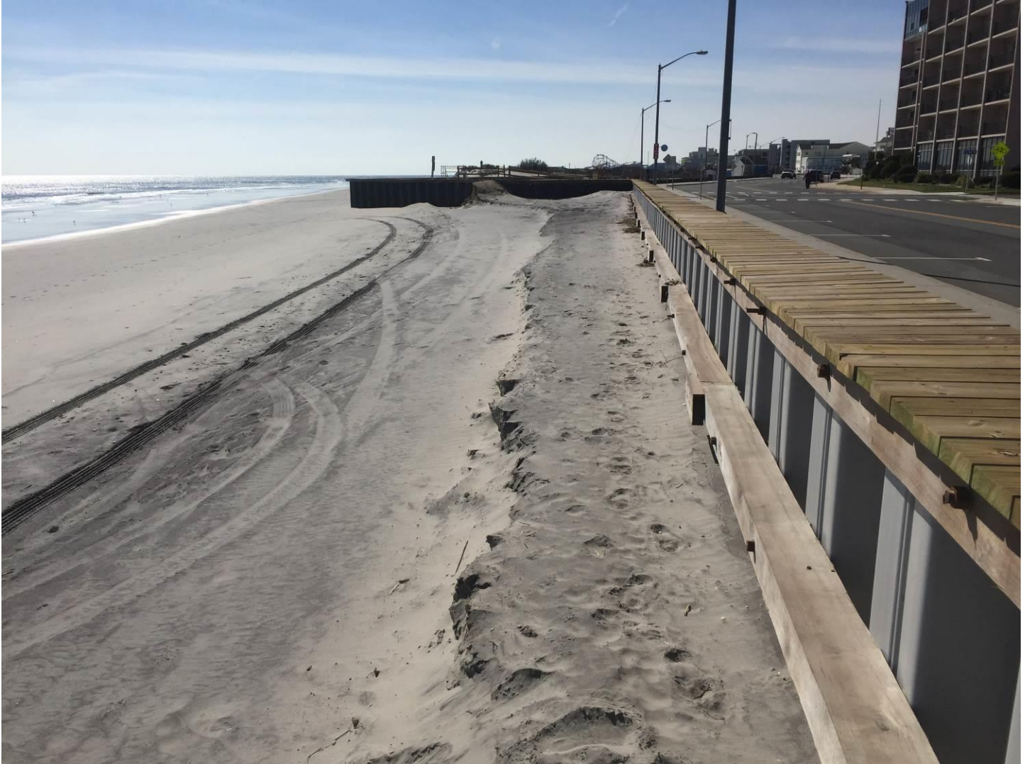
Figure 13. View to the south taken from directly in front of the cap on the new bulkhead that starts just south of the 3 rd Avenue gazebo on November 5, 2018. The beach is wet almost to the bulkhead as the fall 2018 survey indicates in figure 10 and the sand loss extends 320 feet offshore totaling 28.42 yds 3 /ft. Clearly the sand that has appeared at the inlet jetty at site 00+00 did not arrive by transport north along the shoreline. Sand from this location has moved south generating the losses documented. The 5-foot remnant of the sand back-passed from Wildwood during the late spring of 2018 is all that is left in place from that effort.
