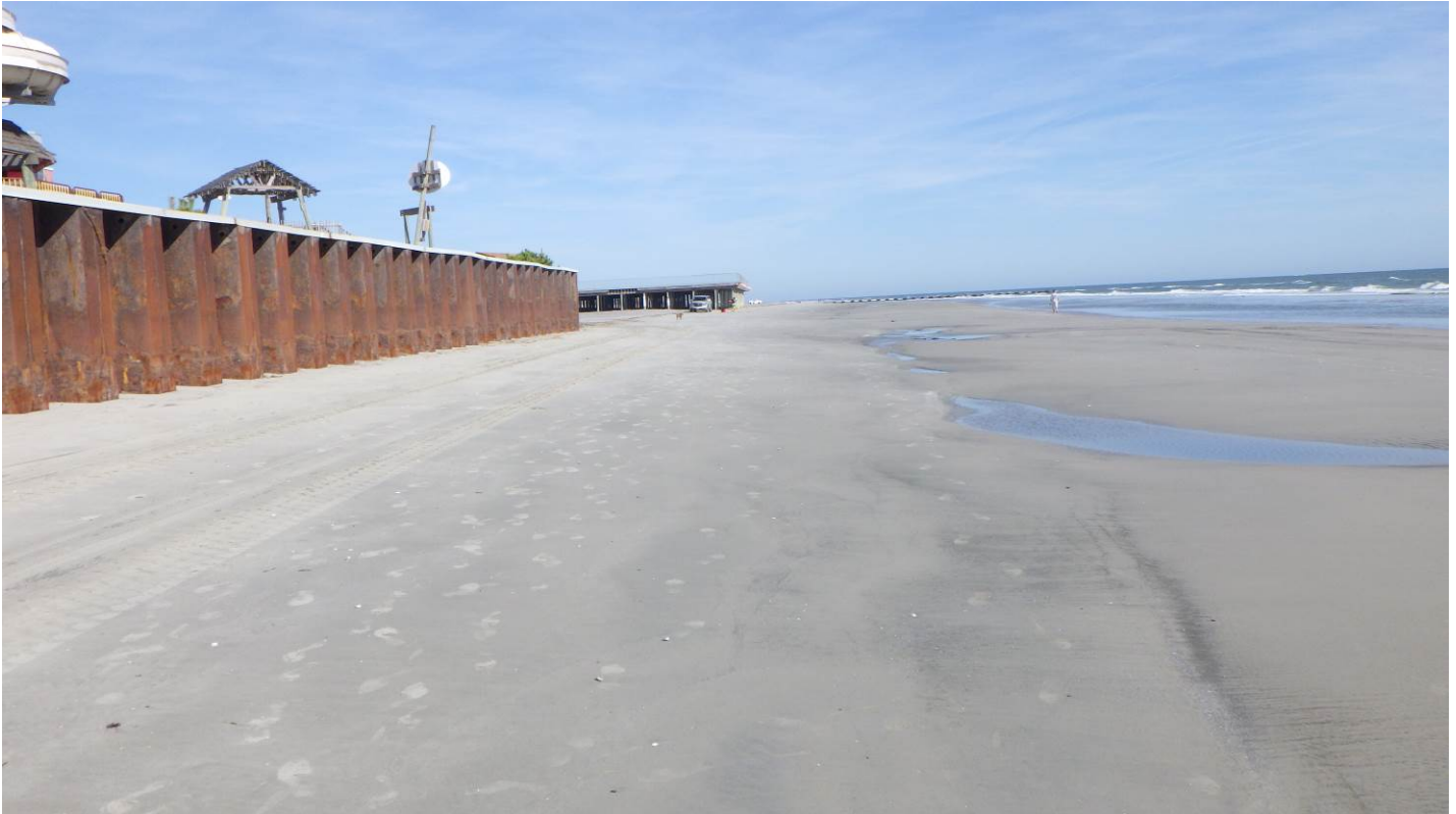
Figure 21. View to the north taken on June 6, 2021 seaward of Morey's Surfside Pier with the steel bulkhead protection positioned just at the last high tide mark indicated by the plant debris at the foot of the bulkhead. This is not a beach where shore protection is significant. The gradient is relatively flat as can be seen looking toward the timber pier in the distance.
